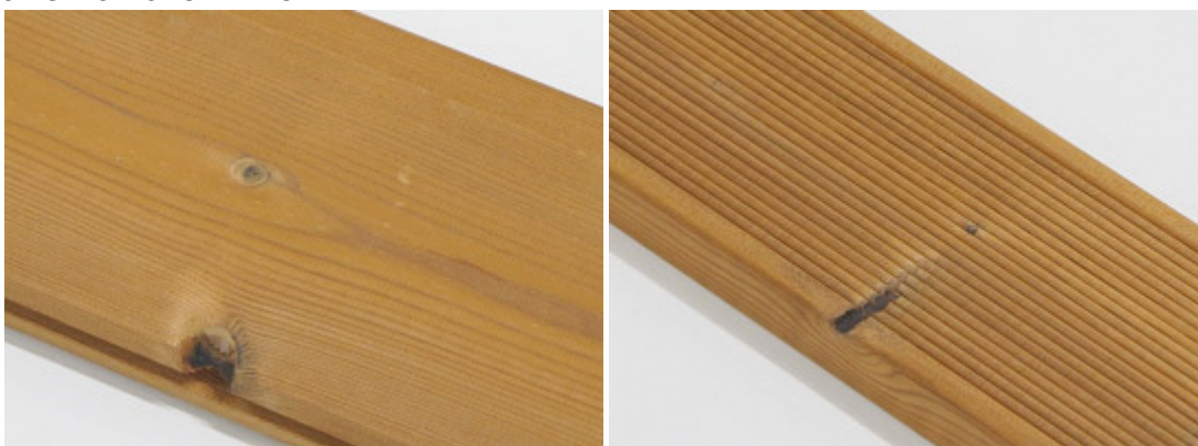
SMALL MISSING KNOT ON THE EDGE
