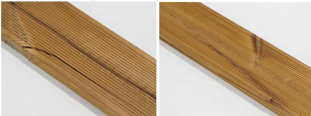
SEVERE SHAKES AND CRACKS
